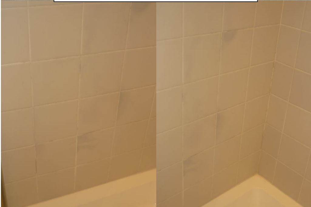
Dark stain marks to walls in shower unit in Bathroom
